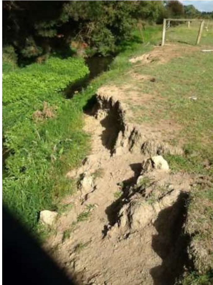
Figure 10 Over steepened banks can erode by dry ravel, South Brook above Buckleys Road at R22-23 (ECan streamwalk)
