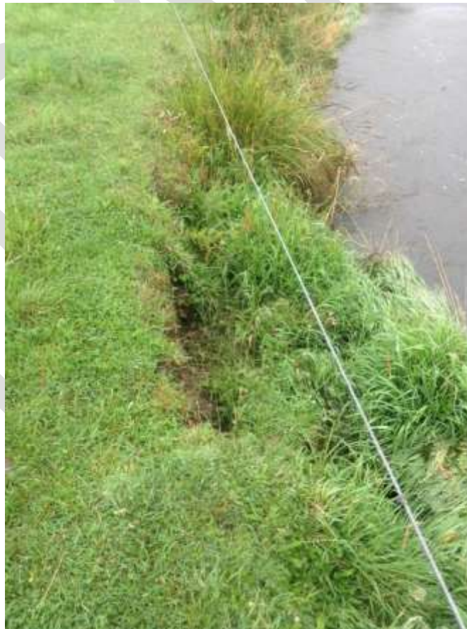
Figure 9 Toe scour and collapse, North Brook above Marsh Road at R4 in Figure A3: 2A (ECan streamwalk)
